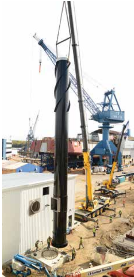
The stack for the Boiler Building is shown during installation on October 15. Photo by G. Hilt.
